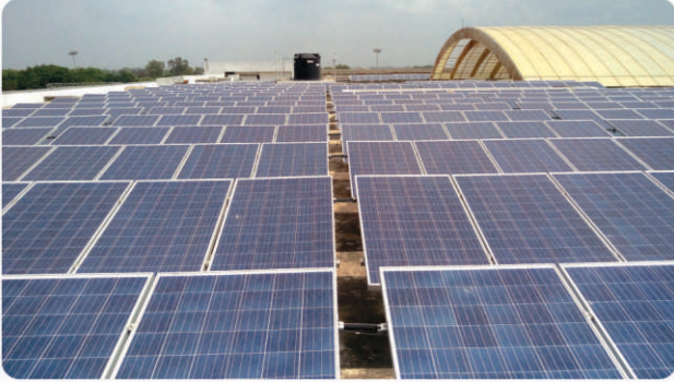
720KW Solar Power Plant Ahmedabad Airport - Airport Authority of India
