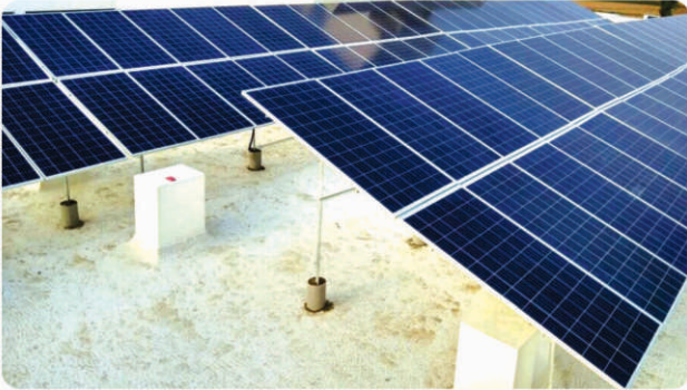
50KW Solar Power Plant Anand Niketan - Maninagar
